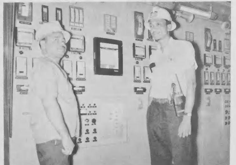
Employees also in charge of "Tosi" boiler startup for HDS are (l) M. Croes, operator, and J. Bishop, shift foreman. Not in picture are: C. B. Geerman and D. Perez.
